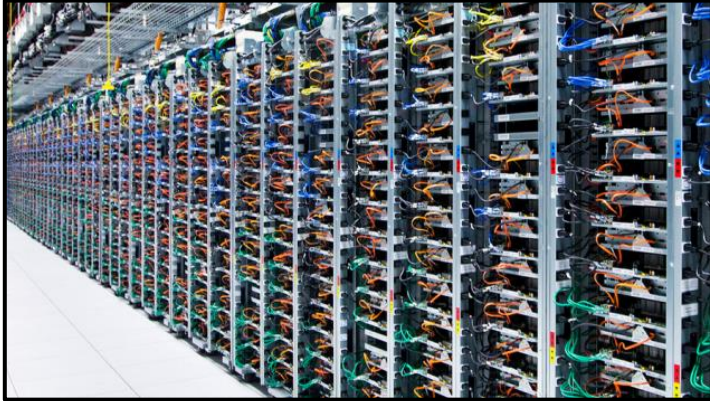
Next-Generation Datacenter Cluster
